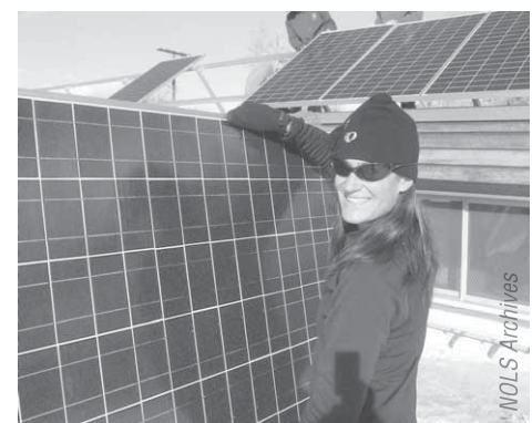
The newly installed solar panels at NOLS Rocky Mountain are an example of the Environmental Stewardship goal in action.
