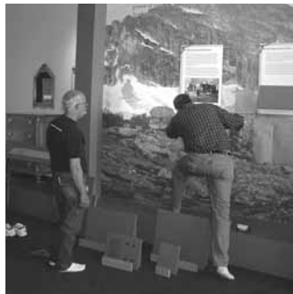
The renovated gallery space (top photo) is transformed as workers install exhibits (bottom photo).
